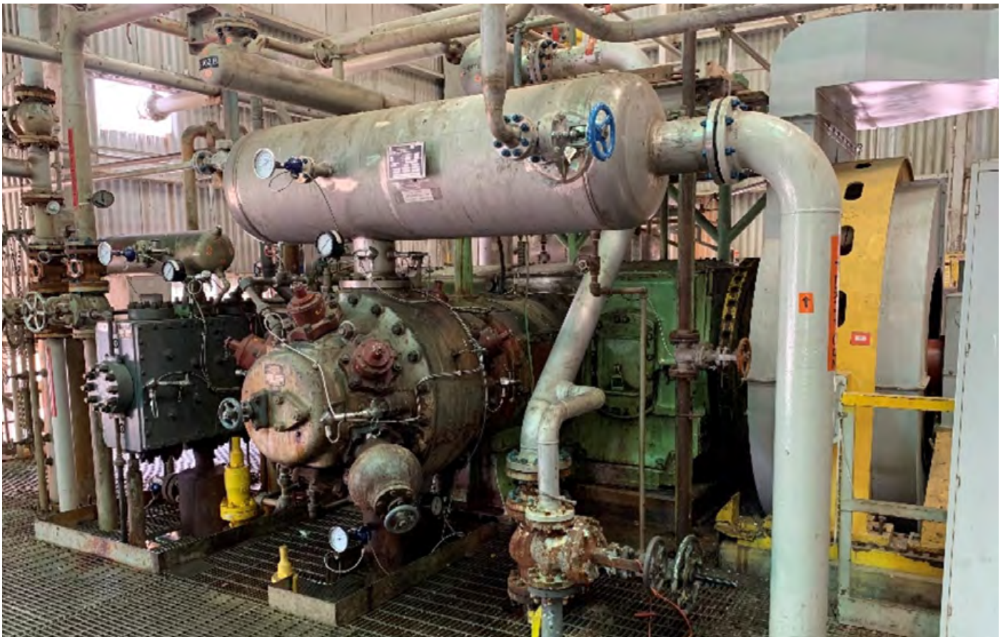
Figure 1. One of the two CO 2 reciprocating compressors used in the ammonium carbamate process.
