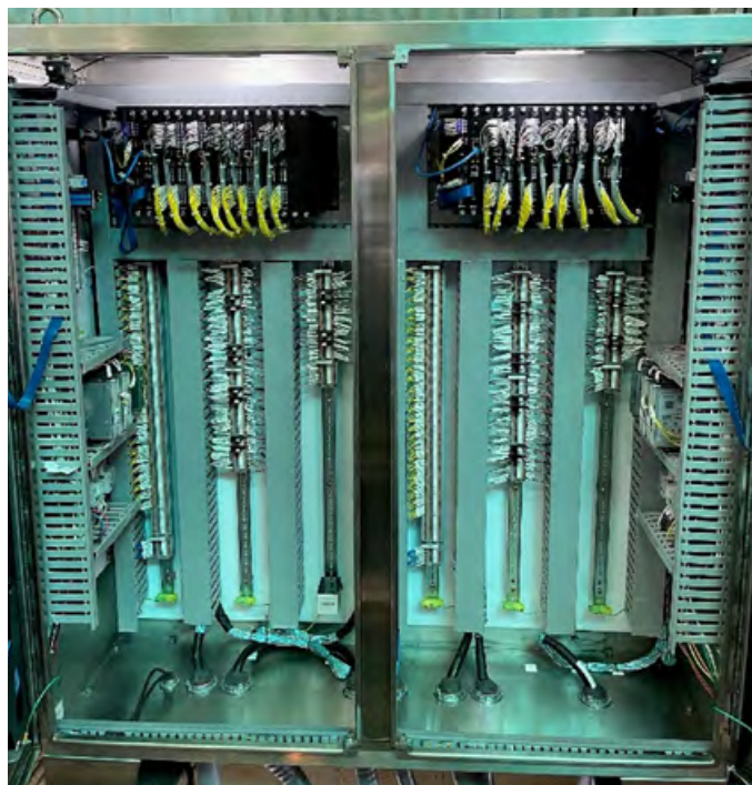
Figure 2. Rear view of the two VC-8000 monitoring racks mounted in the cabinet.
